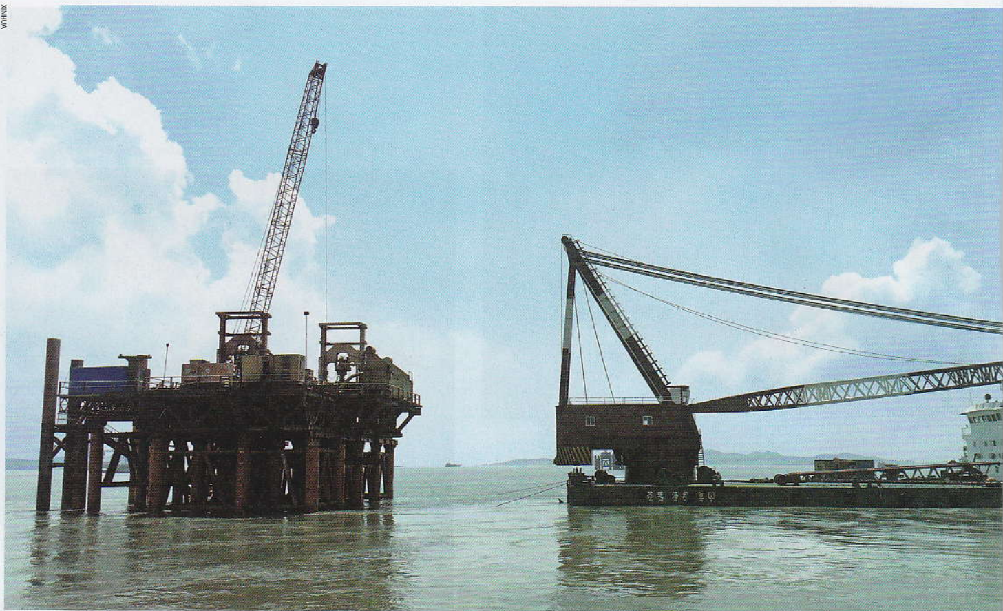
Construction is underway to install super large wind turbines in Xinghua Bay, Fuqing, Fujian Province, on August 25
